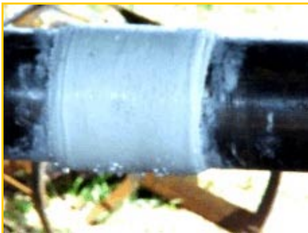
Figure No. 17 - Failed @ 2,000 psi
