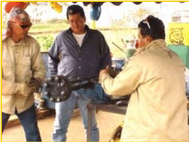
Figure No.1 -Cleaning to White Metal the Repair Area for Defect "A"
